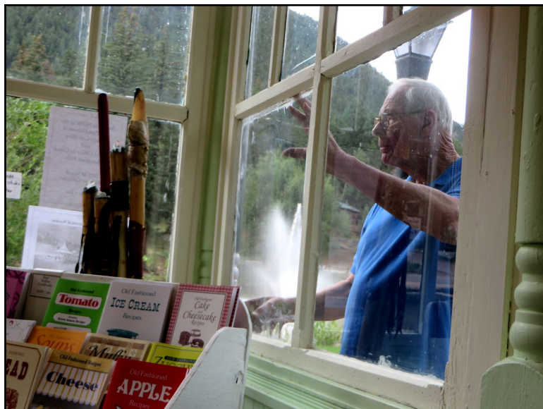
Volunteer Joe Olds finishing up repairs on the Land Office Photo by Judy Perkins
